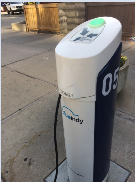
A BlueIndy charging station | © RTO Insider
