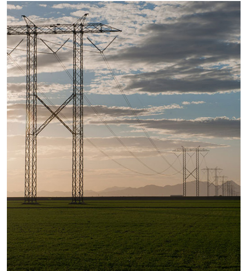
Transmission lines near Blythe, Calif. | U.S. Bureau of Reclamation
