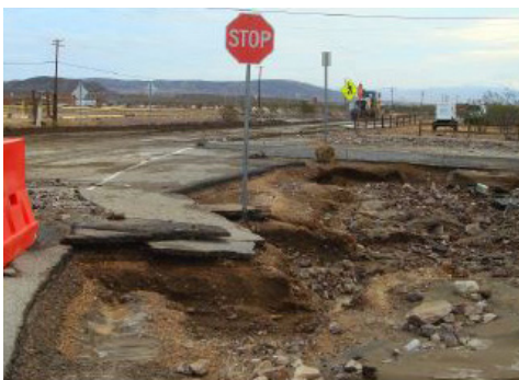
In 2013, Fort Irwin, Calif., experienced three power outages within 45 days as a result of flash floods from extreme rain events | U.S. Army
