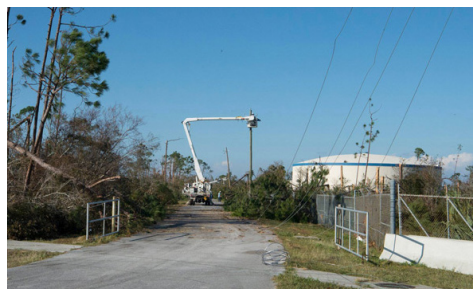
Crews repair power lines at Tyndall Air Force Base after Hurricane Michael hit the Florida Panhandle in October. | U.S. Air Force
