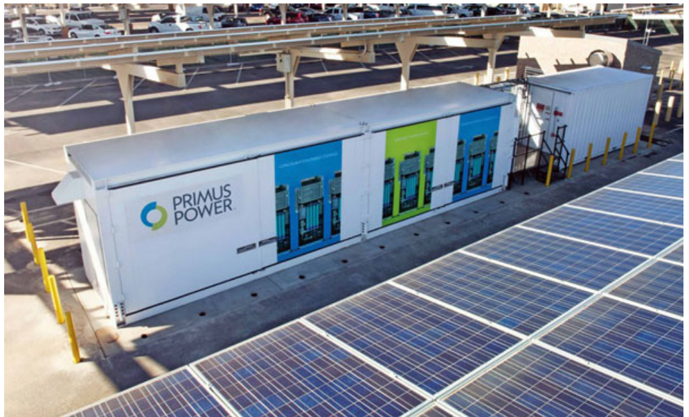
Marine Corps Air Station Miramar has a microgrid powered by landfill gas, solar energy, storage, diesel generation and natural gas that can power the installation for three weeks. | U.S. Marine Corps
