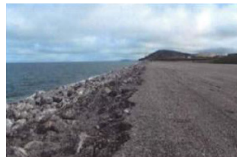
The Air Force spent $46.8 million to repair erosion to the rock seawall at the Cape Lisburne Long Range Radar Station, Alaska, which protects its airstrip from waves. | U.S. Air Force
