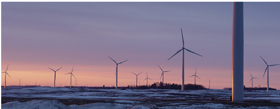
Fenton Wind Farm near Chandler, Minn.
