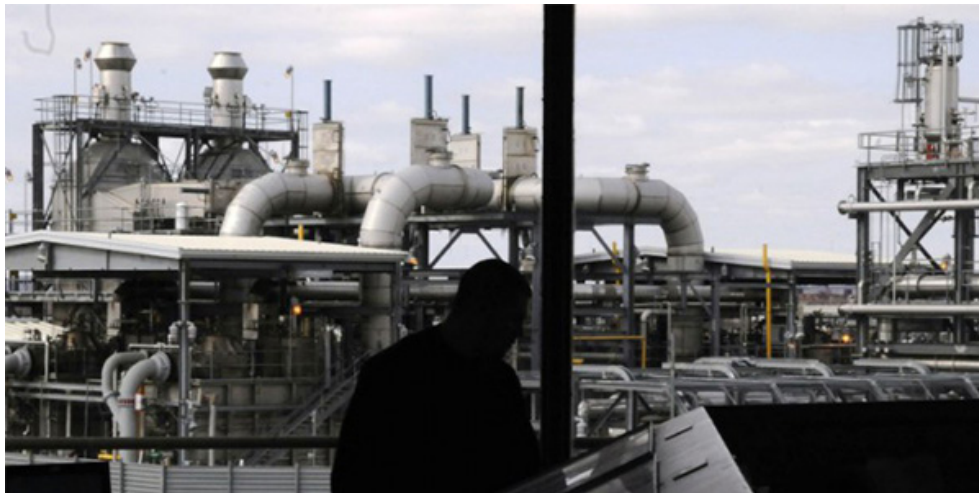
View from the control room at Exelon's Distrigas LNG terminal in Everett, Mass. | ENGIE
