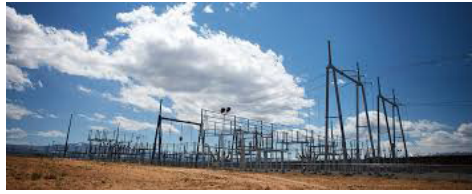
Tri-State G&T transmission upgrade project in Colorado | Tri-State G&T
