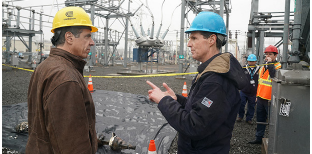
Con Edison CEO John McAvoy (right) leads New York Gov. Andrew M. Cuomo on a tour of a substation in Astoria Queens where an electrical fault on 138,000-volt equipment caused a sustained electrical arc flash visible across a wide area of the city on Dec. 27. Cuomo asked state regulators to investigate the incident, which disrupted operations at LaGuardia Airport and a nearby subway line. | Gov. Cuomo
