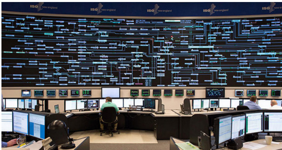
ISO-NE control room | ISO-NE
