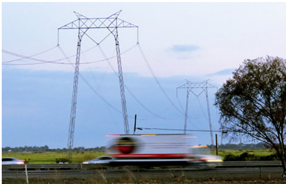
A major PG&E transmission line crosses Interstate 80 near Sacramento. | © RTO Insider
