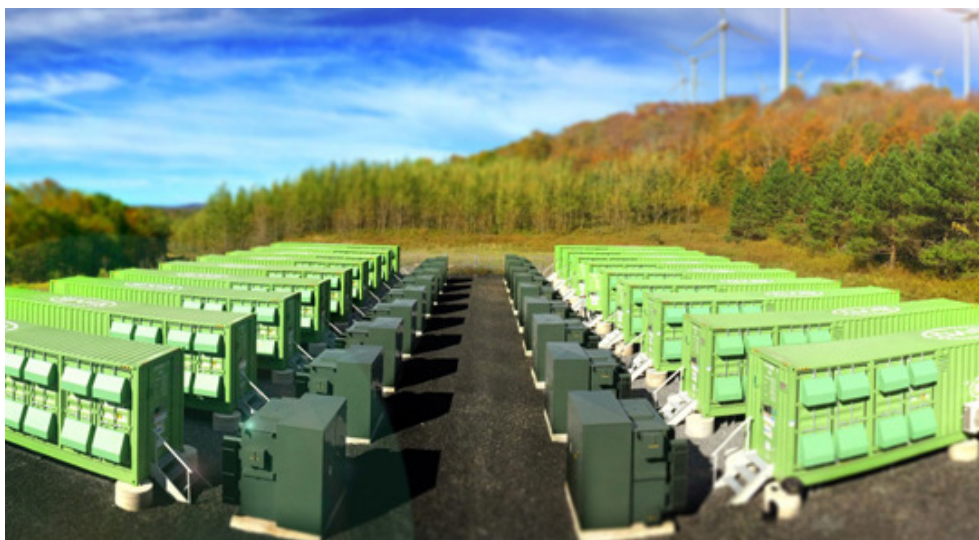
Invenergy's 31.5-MW Grand Ridge Energy Storage project | Invenergy
