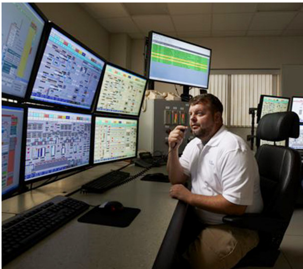
The control room at Duke Energy’s Buck combined cycle plant in Rowan County, N.C. | Duke Energy
