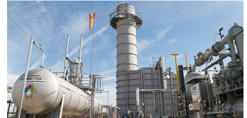
A Southern California Edison natural gas peaker plant near Los Angeles | SCE
