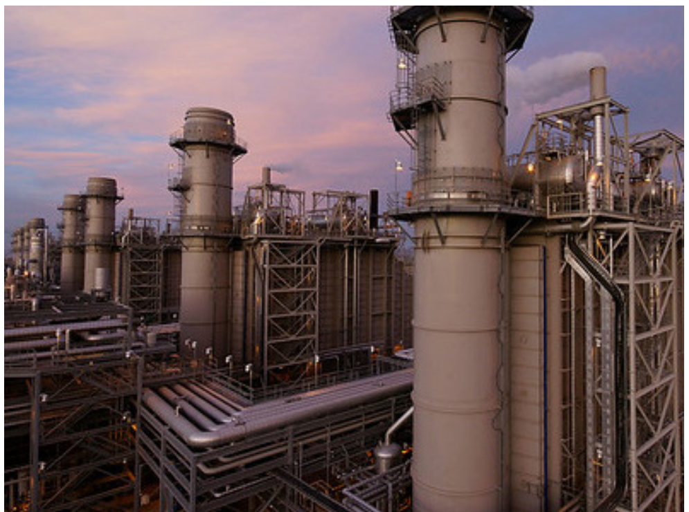
Gila River Power Station | SRP
