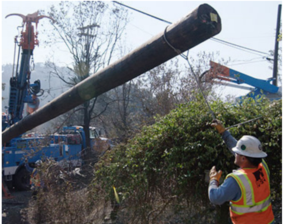
PG&E's wildfire mitigation plan includes enhanced vegetation management around power lines. | PG&E
