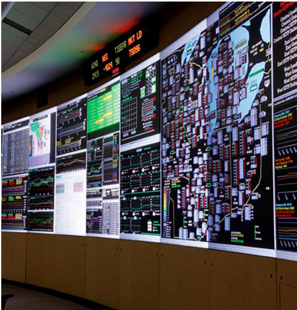
MISO control room | MISO
