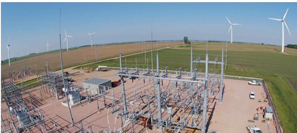
Xcel Energy upgrade project | Burns & McDonnell
