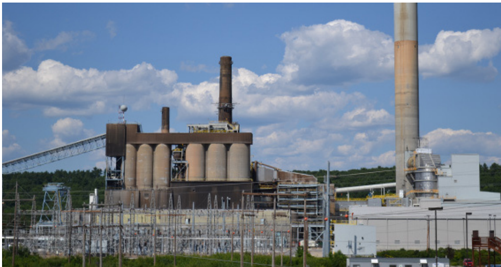
The 440-MW Merrimack Station in Bow, N.H., is New England's largest remaining coal-fired power plant.
