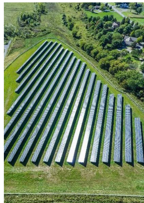
A 2-MW solar project at Mohawk Valley Community College was supported by a grant from the New York State Energy Research and Development Authority. | NYSERDA
