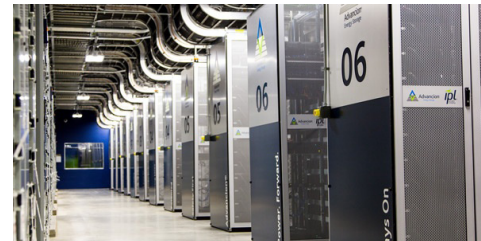
Harding Street Energy Storage in MISO | AES
