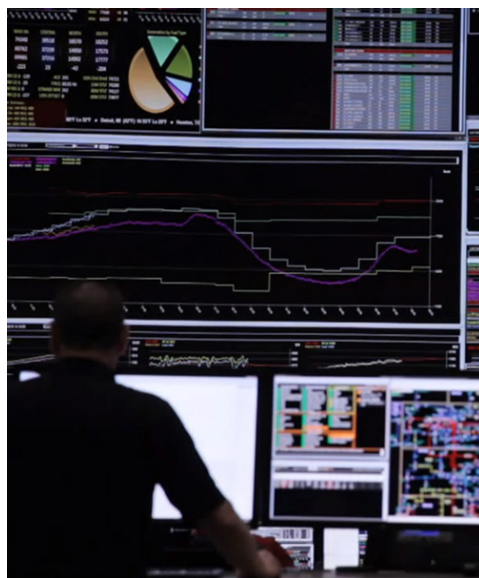
MISO control room | MISO
