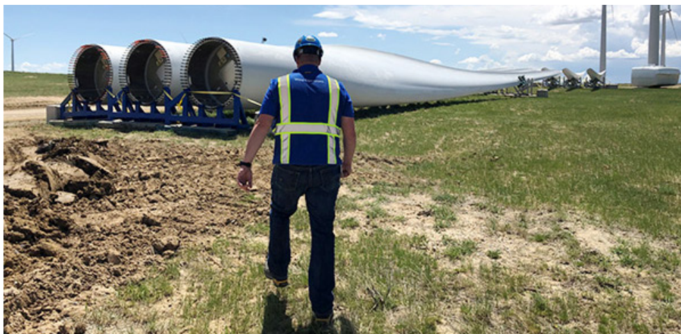
Part of Rocky Mountain Power's Energy Vision 2020 plan is repowering wind turbines at its Seven Mile Wind Farm with longer blades. | © RTO Insider
