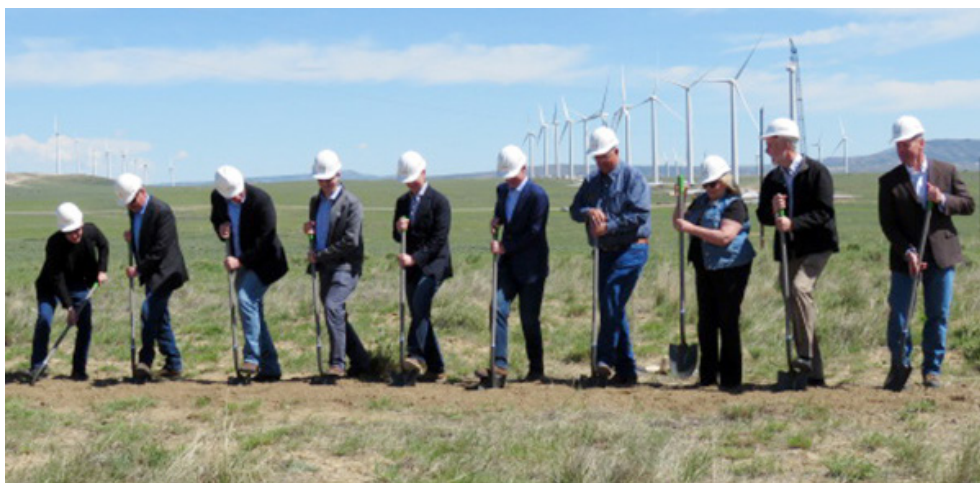
Executives with Rocky Mountain Power broke ground on 1,150 MW of new wind power June 5. | © RTO Insider
