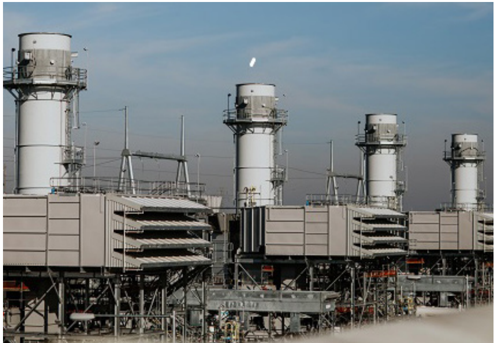
OG&E's Mustang Energy Center features gas-fired quick-start units. | OG&E
