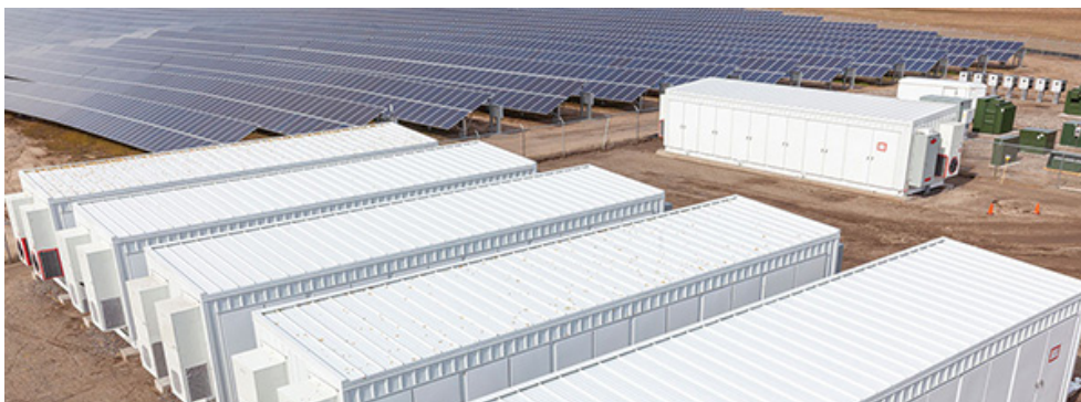
Energy storage in Minnesota | Connexus Energy
