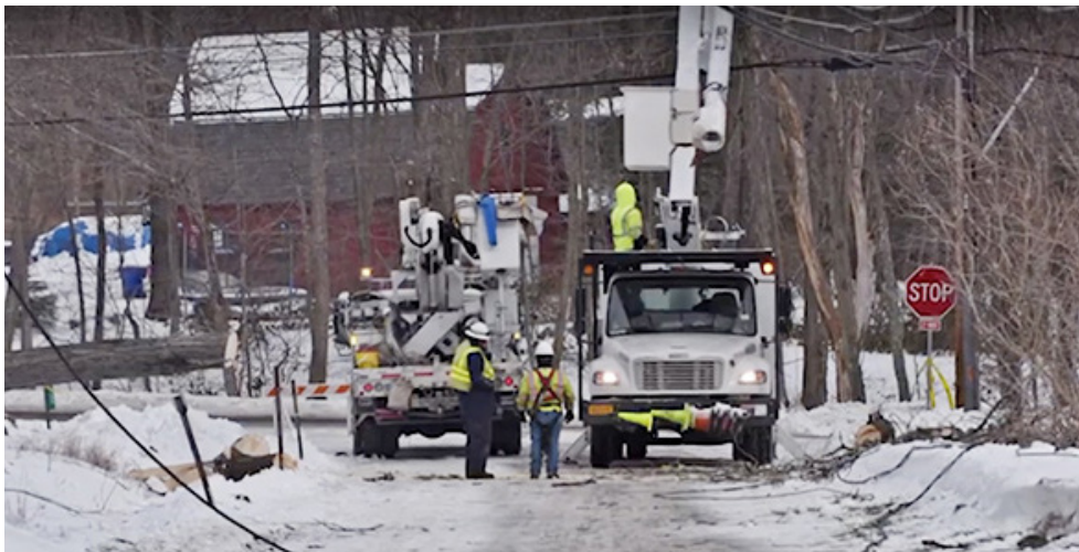
Eversource crews work to restore power following a Jan. 20 ice storm in Connecticut. | Eversource Energy
