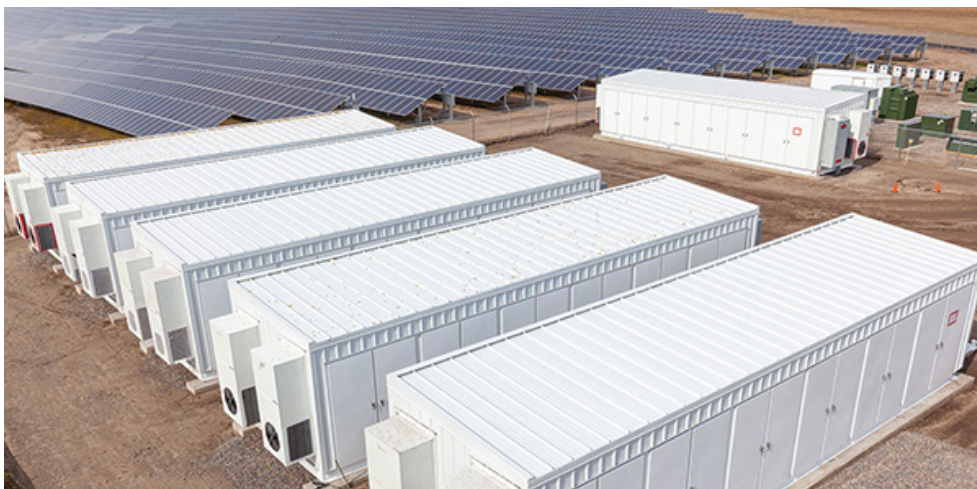
Energy storage in Minnesota | Connexus Energy
