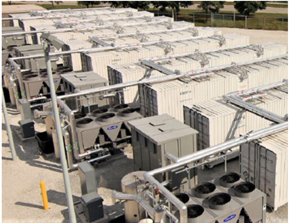
AES battery storage | AES
