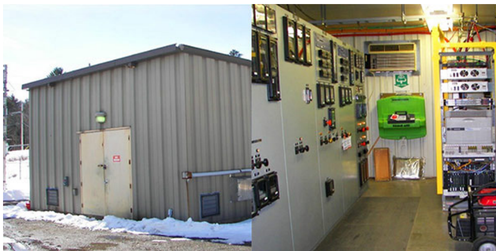
VELCO's Berlin substation control building lacks space to accommodate needed improvements, communication equipment and ancillary systems. | VELCO
