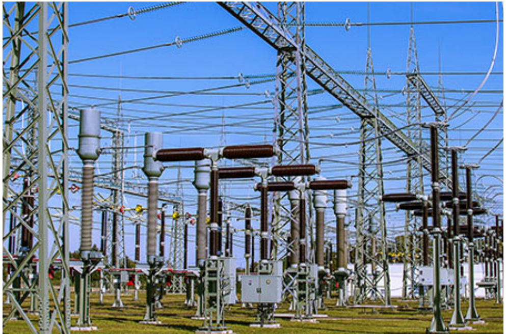
A TO-proposed Tariff filing that skirts FERC-ordered transparency rules for replacing certain critical substations left other stakeholder sectors uneasy last week. | Pexels
