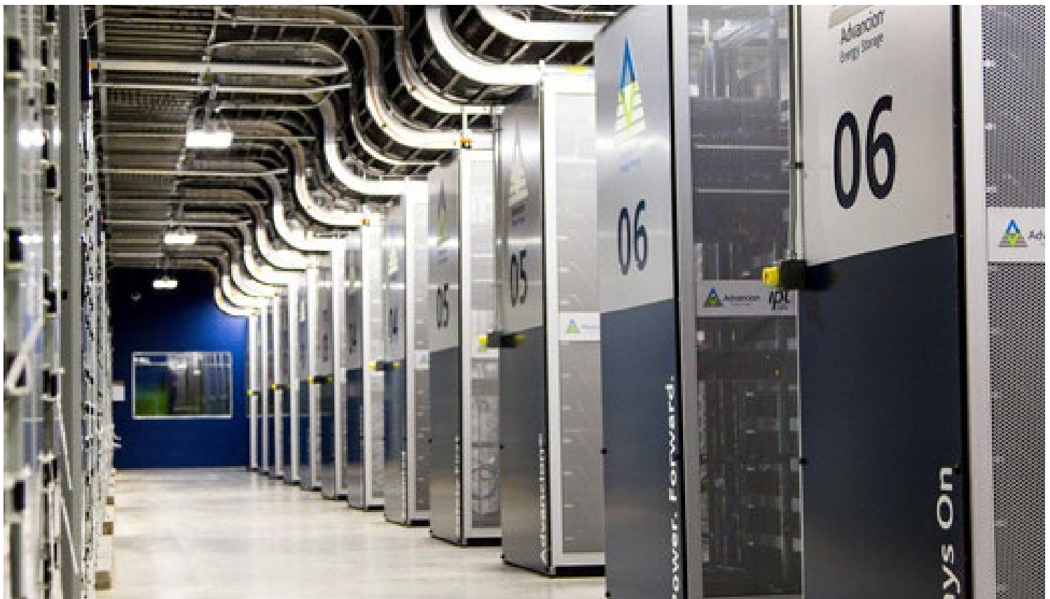
Harding Street Energy Storage in MISO | AES
