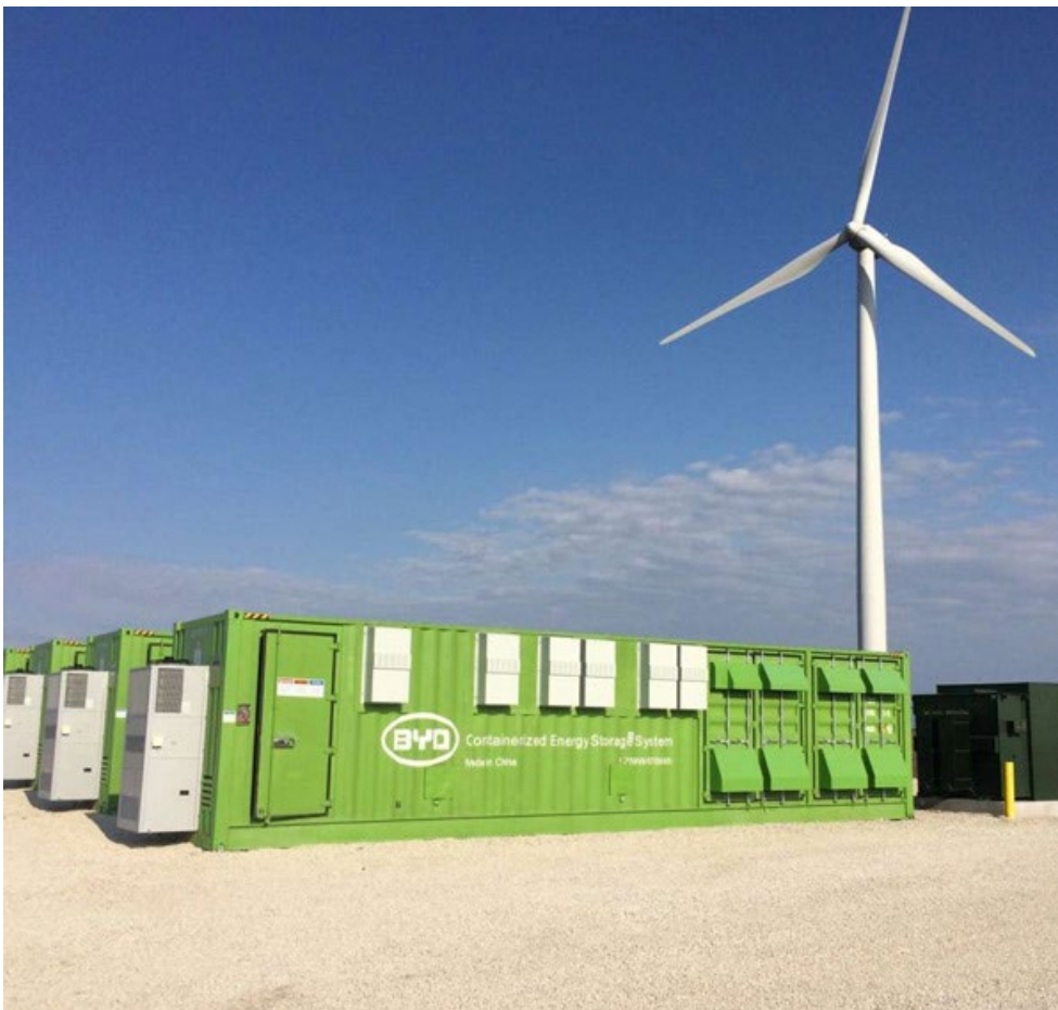
Invernergy's Grand Ridge Battery Storage Facility in Illinois | BYD
