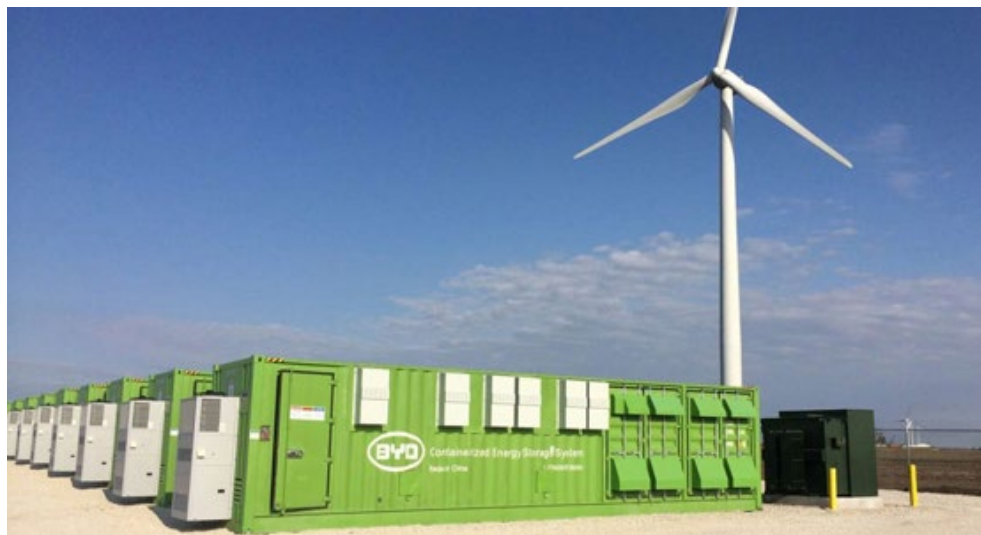
Invenery's Grand Ridge Battery Storage Facility in Illinois | BYD
