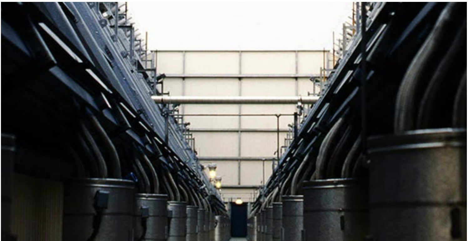
Combined cycle generator at Doswell Energy Center | Fluor
