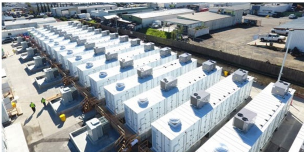
San Diego Gas & Electric's 30-MW battery energy storage facility in Escondido, Calif. | SDG&E
