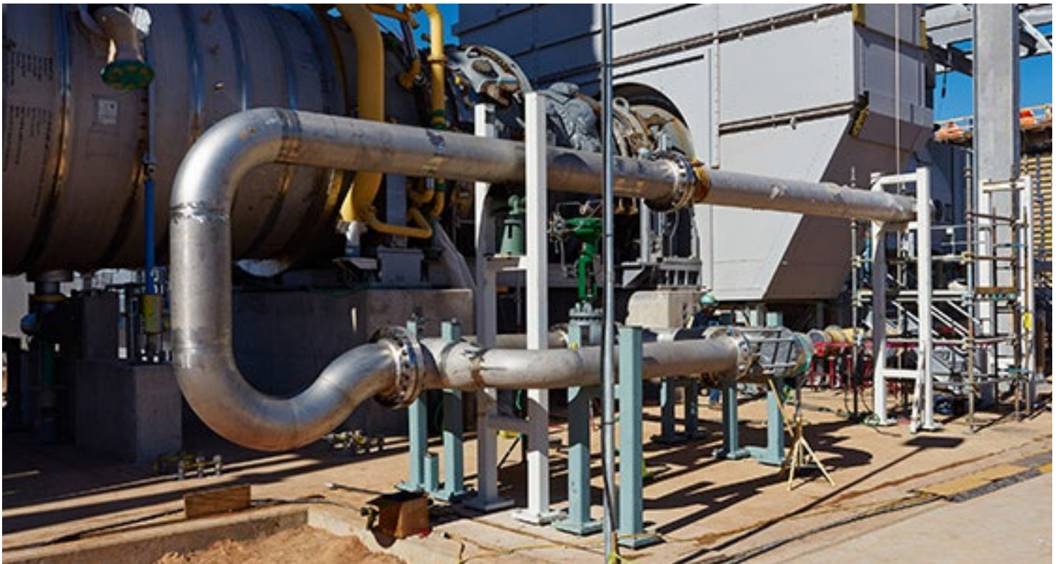
Gas turbine at Golden Spread’s Elk Station plant | GE
