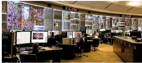
MISO control room | MISO
