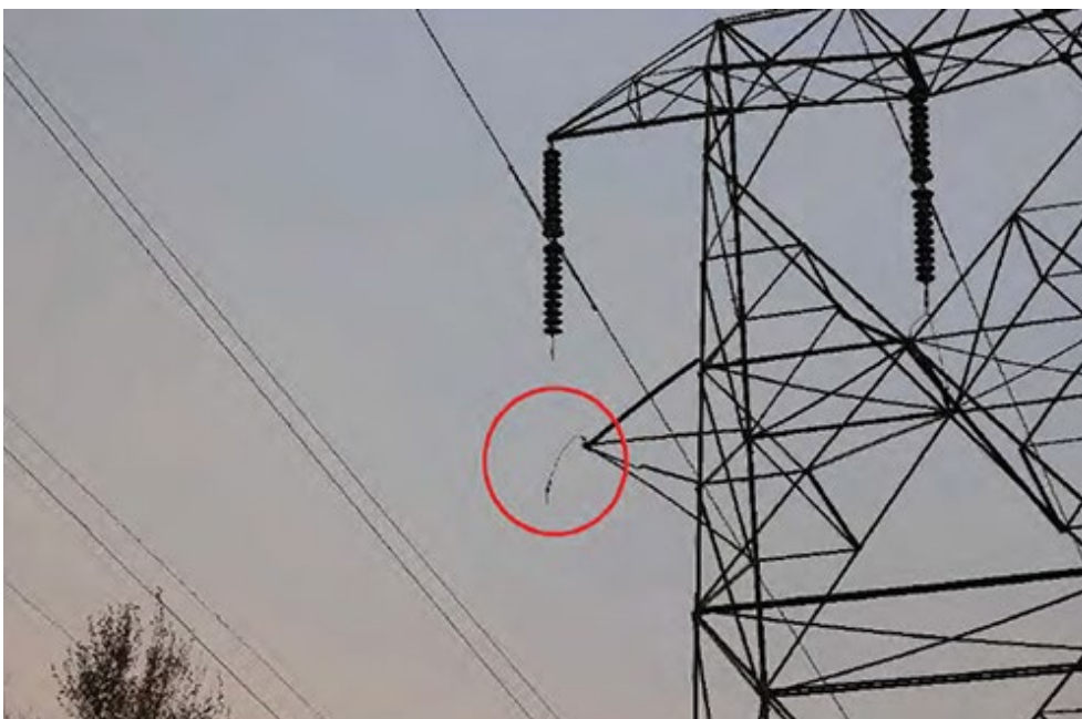
On the tower suspected of starting the Camp Fire in November 2018, an insulator detached from the hangar plate and hung upside down. | PG&E/CPUC
