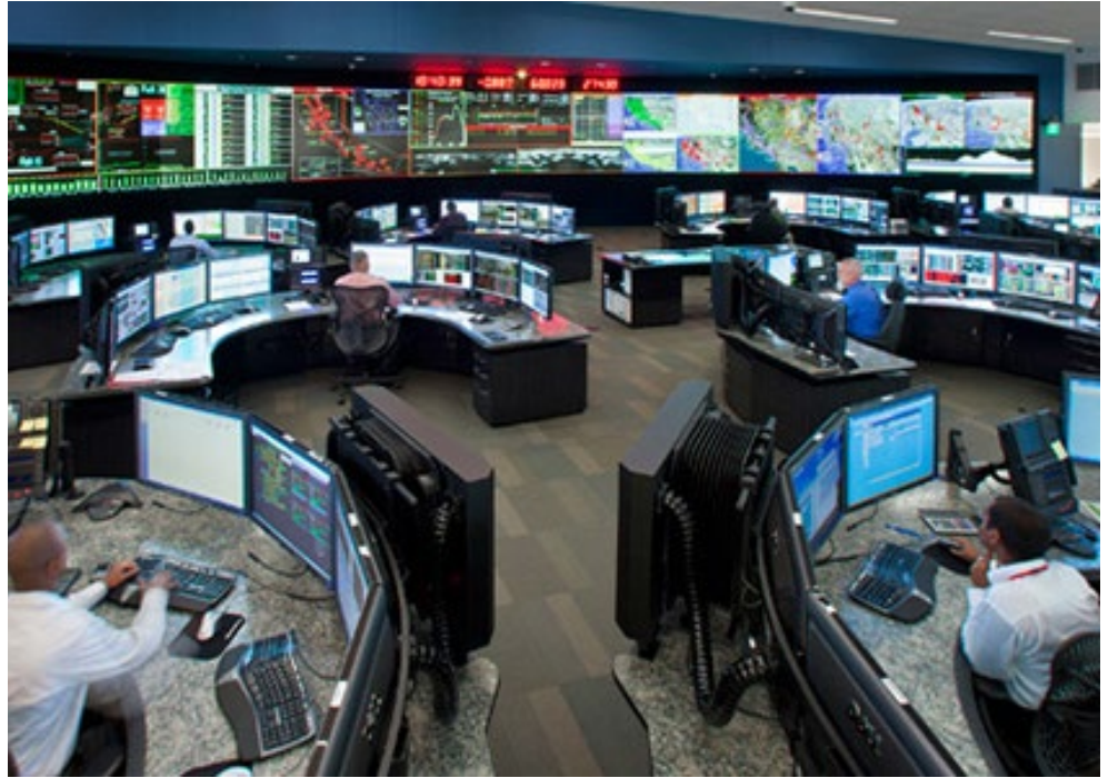
CAISO's control room in Folsom, Calif. | CAISO
