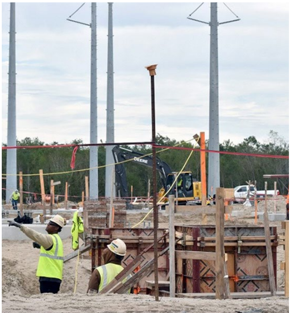
Entergy Louisiana crews work in November on new lines and a substation near the Jefferson and Plaquemines Parishes. The $100 million reliability project is slated for completion in mid-2020. | Entergy Louisiana
