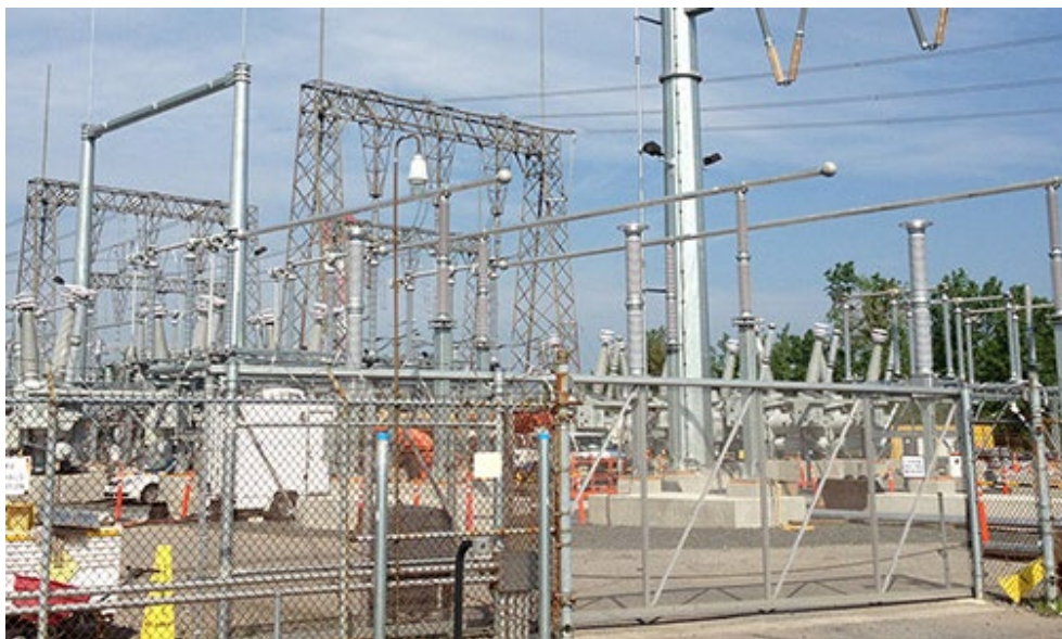
Con Edison's Goethals Substation on Staten Island | Con Edison
