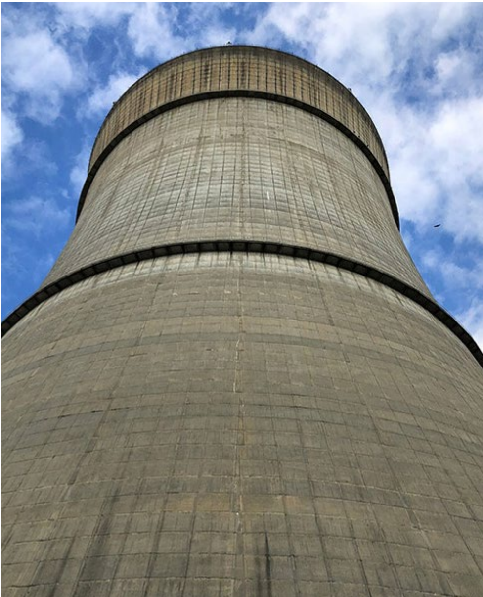
Entergy's Grand Gulf Nuclear Station cooling tower | Entergy Mississippi
