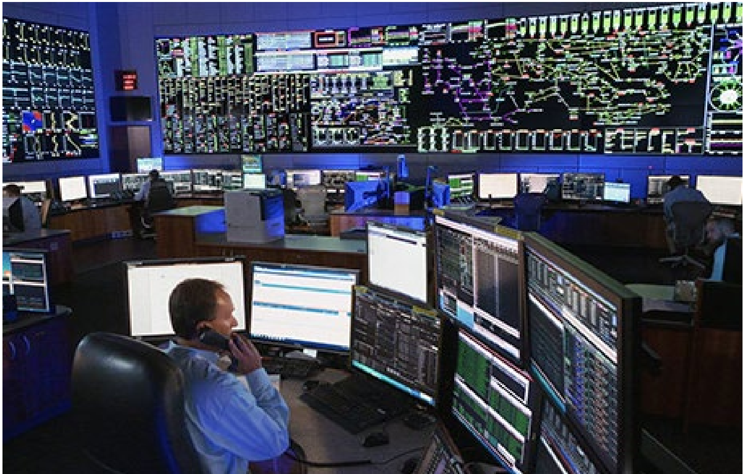
PJM control room | PJM
