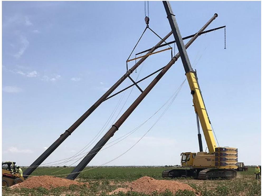
Transmission being built in Xcel subsidiary Southwestern Public Service's territory | SPS
