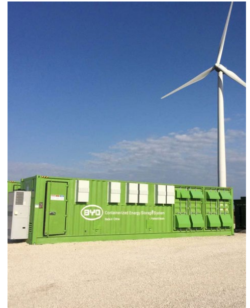
Invenery's Grand Ridge Battery Storage Facility in Illinois | BYD
