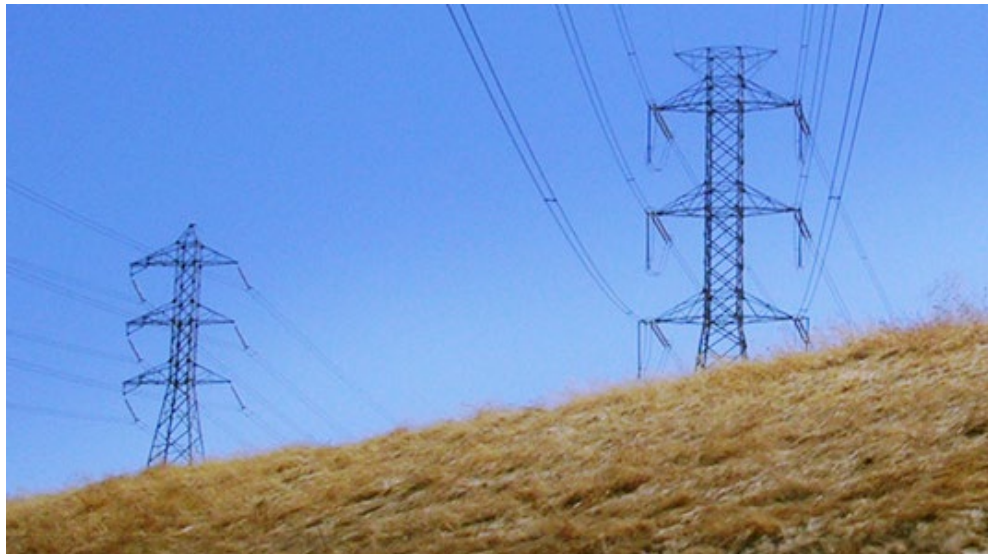
Dual Circuit 500kV power lines
