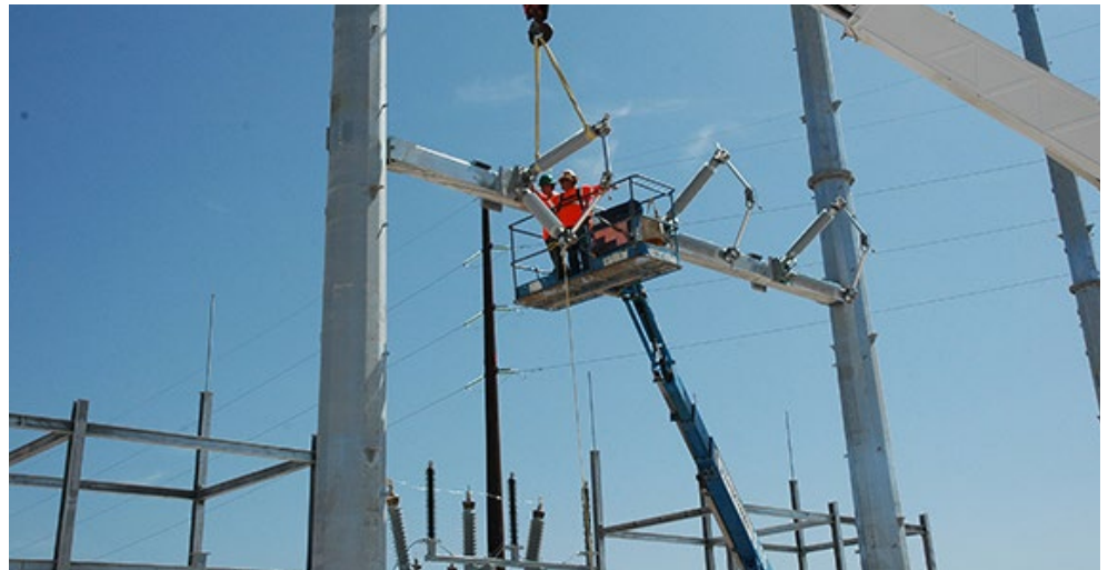
Construction crews work on an SPS substation in New Mexico. | Xcel Energy
