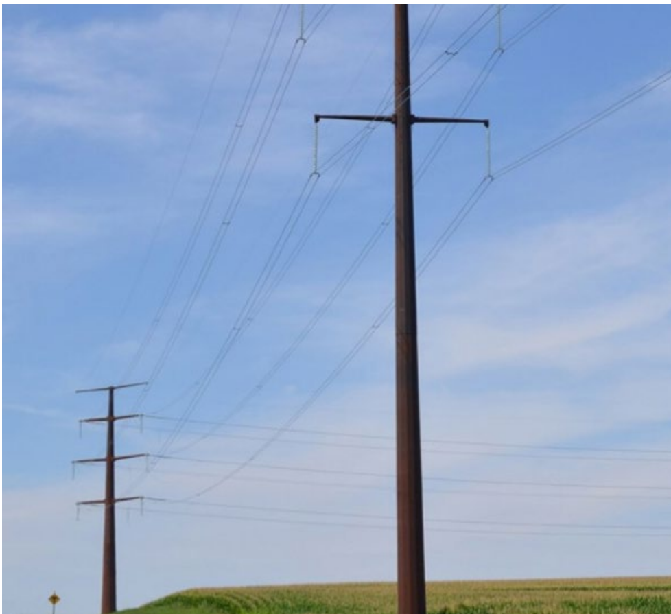
The Brookings County-to-Hampton project, part of CapX2020 | CapX2020
