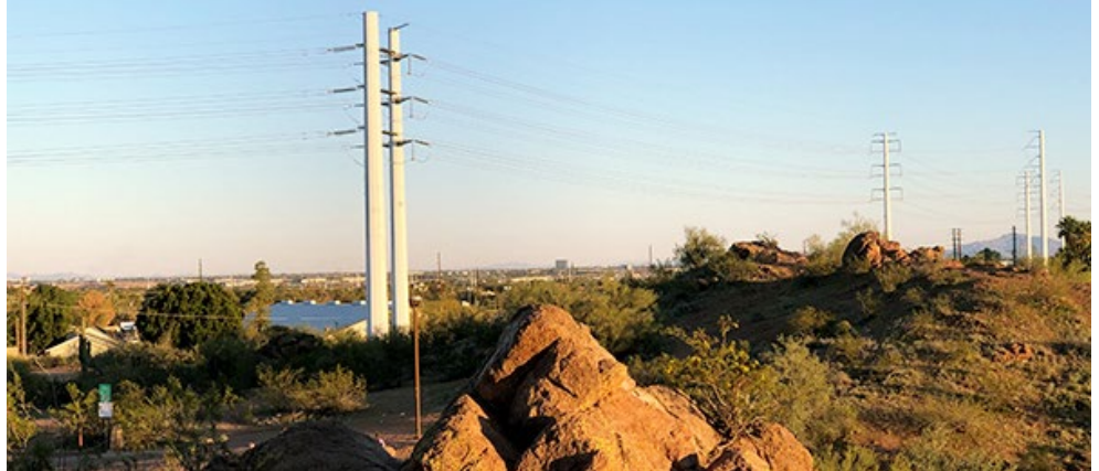
High-voltage lines cross the Salt River Project's PERA Club in suburban Tempe, Ariz., where transmission planners from across the West met Feb. 27. | © RTO Insider
