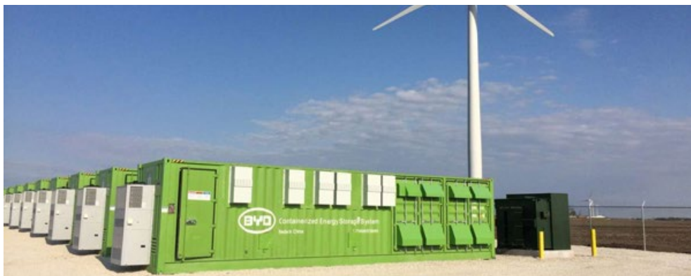
Invenergy's Grand Ridge Battery Storage Facility in Illinois | BYD
