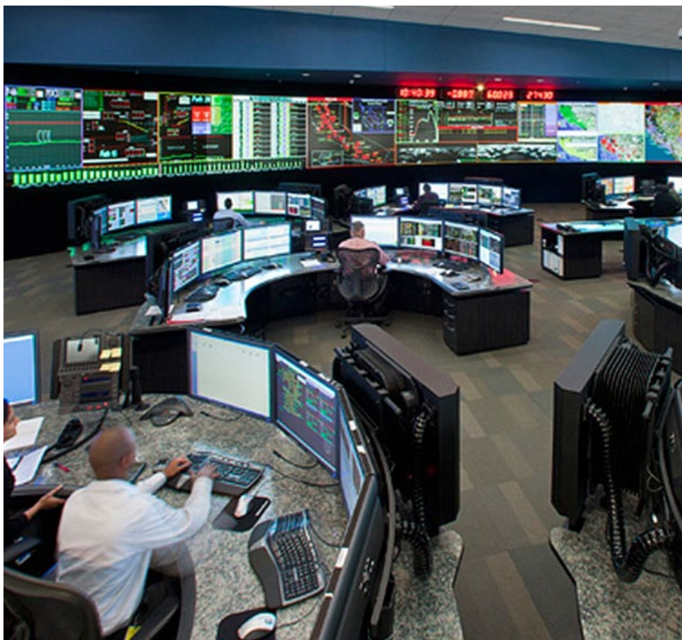
CAISO's Folsom control room | CAISO
