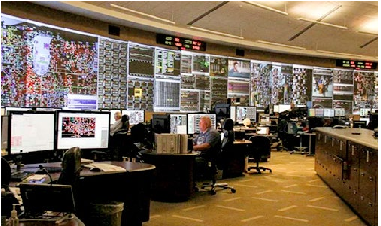
MISO's control room in Carmel, Ind., where the RTO manages pseudo-tie connections. | MISO
