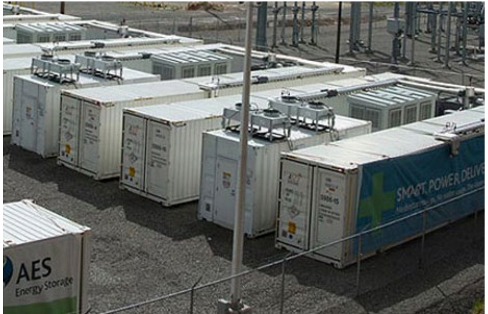
AES' 32-MW Laurel Mountain battery storage project in Elkins, W.Va., is one of the resources covered by the regulation market settlement approved by FERC. | AES
