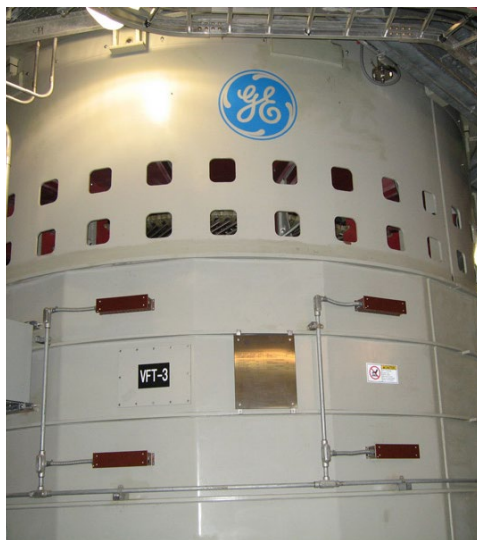
Linden VFT's interior | Energy Initiatives Group
