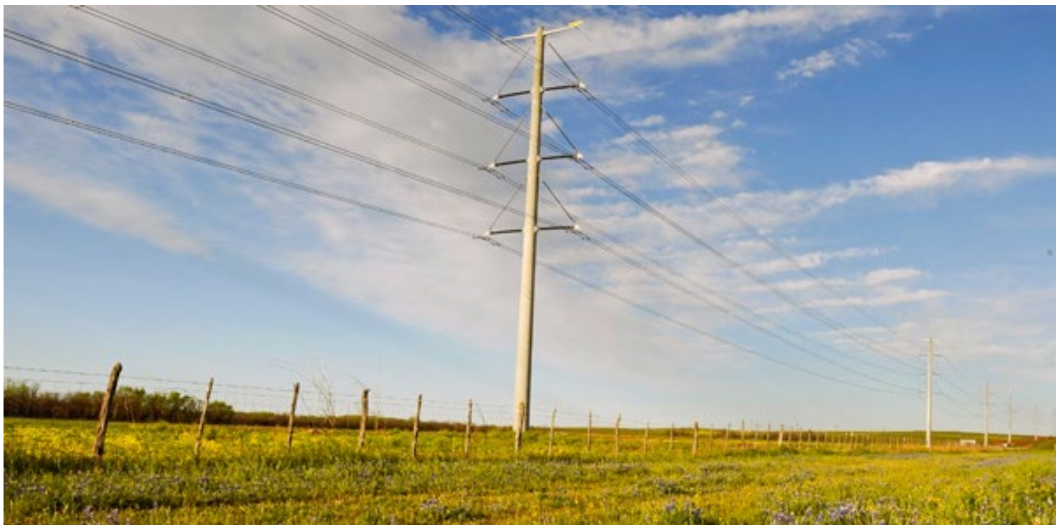
NextEra Energy subsidiary Lone Star Transmission lines | Lone Star Transmission
