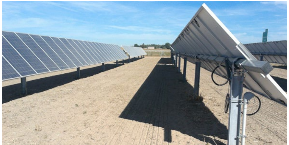
Hoosier Energy Power Network Solar Power Plant in Bloomington, Ind. | Inovateus-Solar
