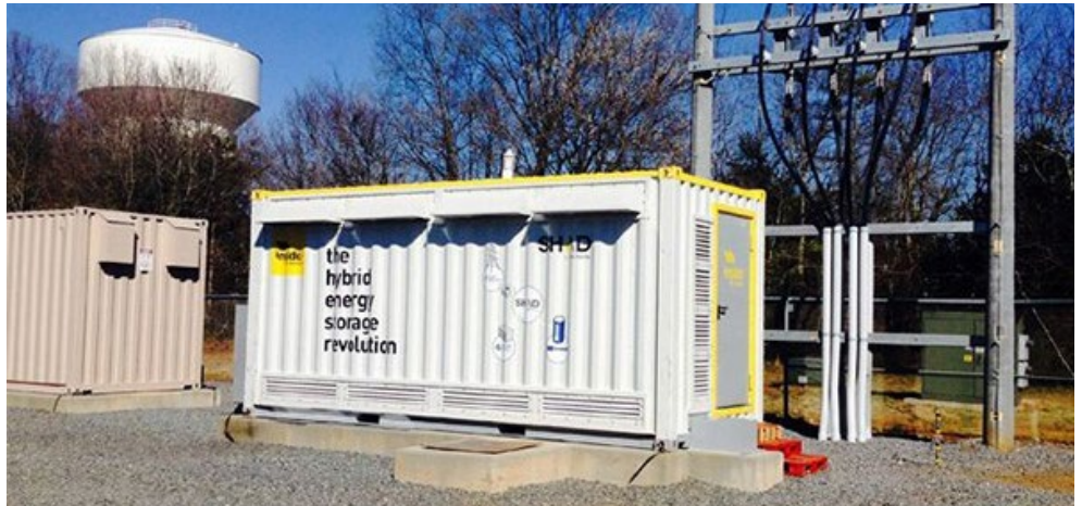
Duke Energy began testing a hybrid ultracapacitor-battery energy storage system (HESS) at its Rankin Substation in Gaston County, N.C., in 2016. The substation is connected to a 1.2-MW solar installation a mile away. | Maxwell Technologies
