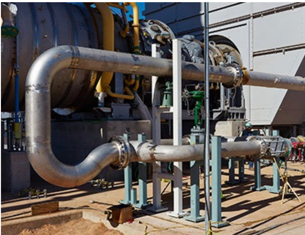
A gas turbine at Golden Spread's Elk Station plant | GE
