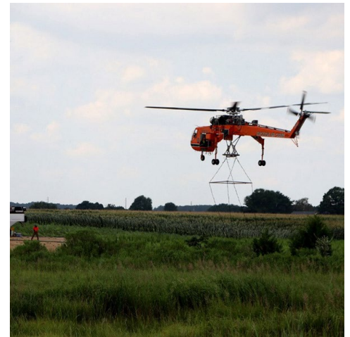
LS Power used helicopters for moving workers and materials during construction of the Artificial Island stability project. | LS Power
