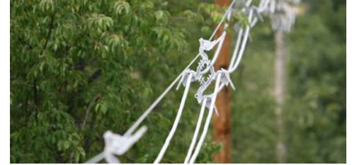
Covered conductor in Southern California is being installed on fiberglass cross arms or in some cases using spacer cable. | SCE
