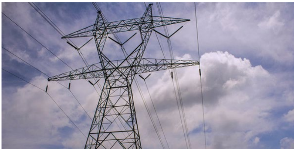
An Entergy transmission tower | Entergy
