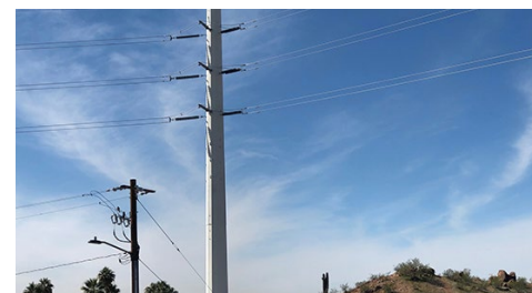
Salt River Project power lines traverse the desert near Tempe, Ariz. | © RTO Insider
