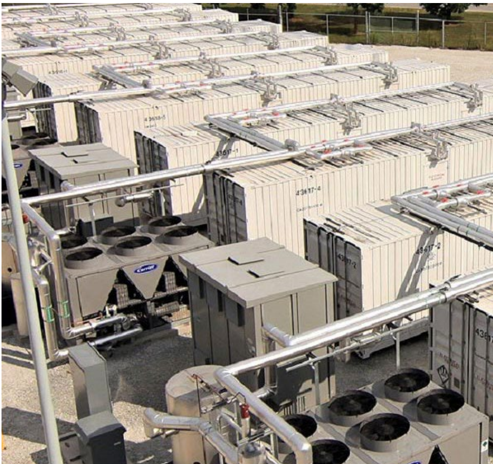
AES battery storage | AES
