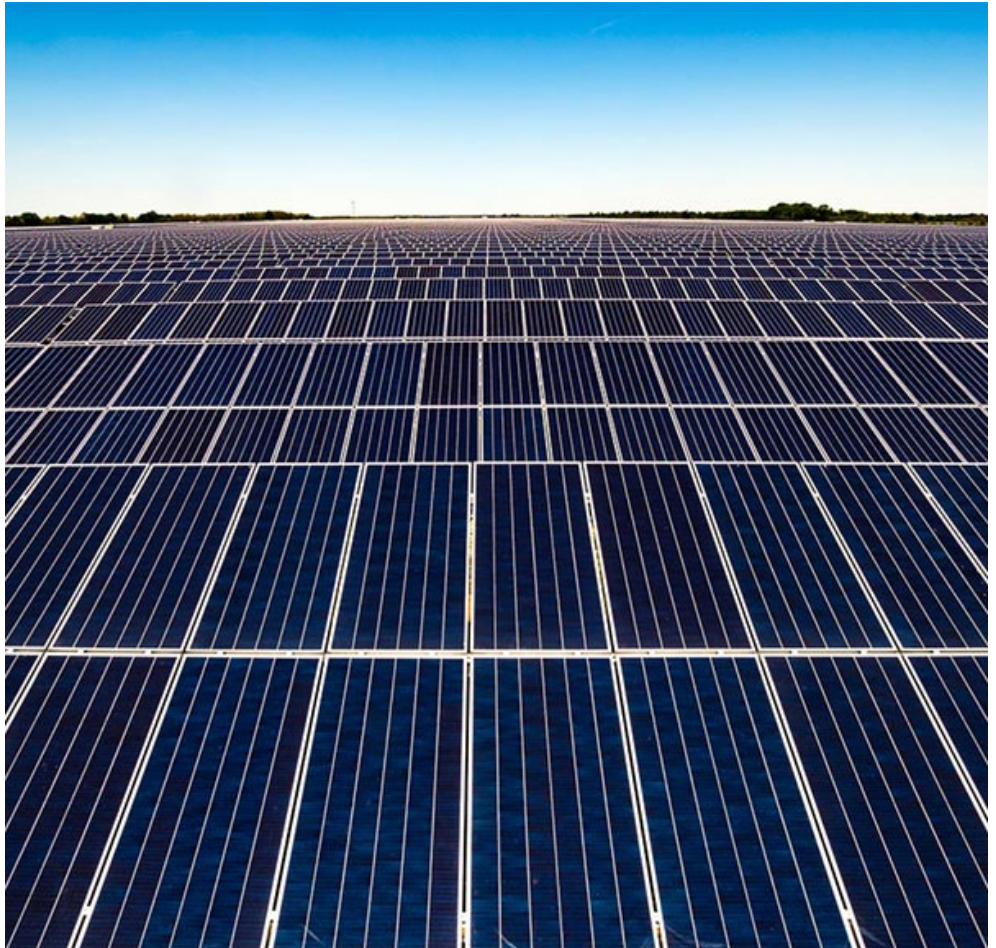
Entergy's Searcy Solar project in Arkansas was one of two 100-MW solar farms recently granted regulatory approval. | Entergy
