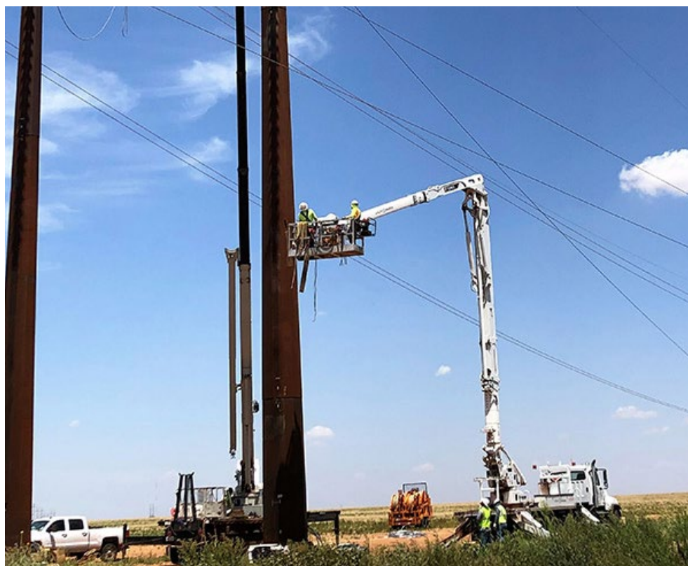
Crews erect an H-frame structure as part of work on the TUCO-China Draw transmission line. | Xcel Energy
