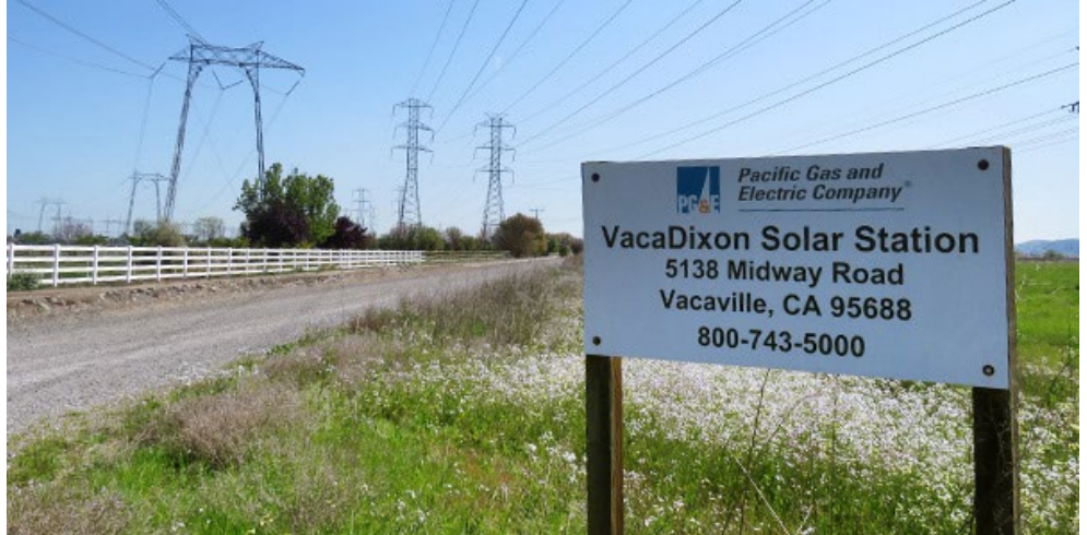
PG&E's VacaDixon solar-and-battery array was the first hybrid resource to participate in CAISO's market starting in 2016. | © RTO Insider
