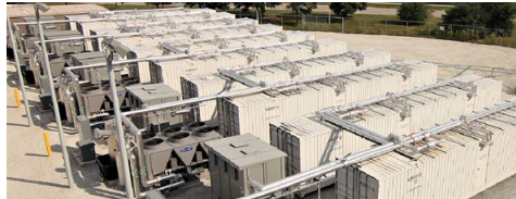
AES battery storage | AES
