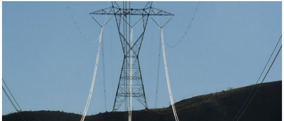
DATC Path 15 transmission line | Duke-American Transmission Co.
