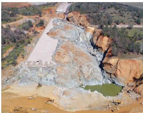
Ultimate damage at the service spillway | California Department of Water Resources
