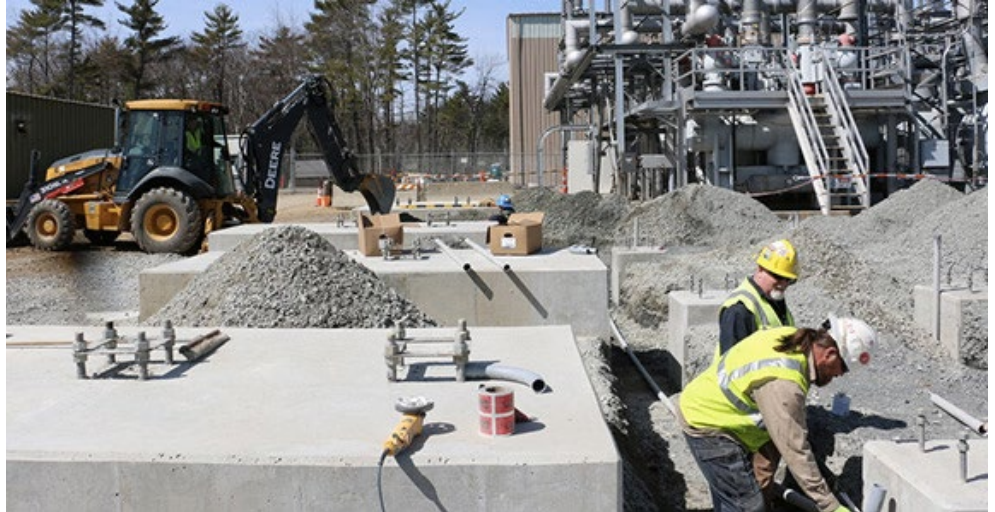
The Tewksbury, Mass., substation is one of three substations involved in National Grid and Eversource Energy's $49 million winning proposal to ISO-NE's Boston 2028 transmission solicitation. | UnitedCivil
