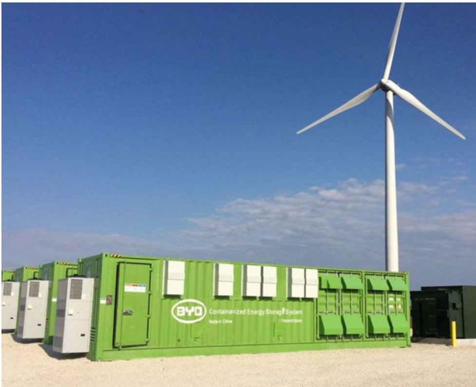
Invenergy's Grand Ridge Battery Storage Facility in Illinois | BYD
