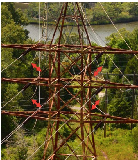
Structure geometry on towers adjacent to the Thames River in Montville, Conn., creates small phase-ground clearances and an increased probability of faults from lightning strikes, according to Eversource. | Eversource
