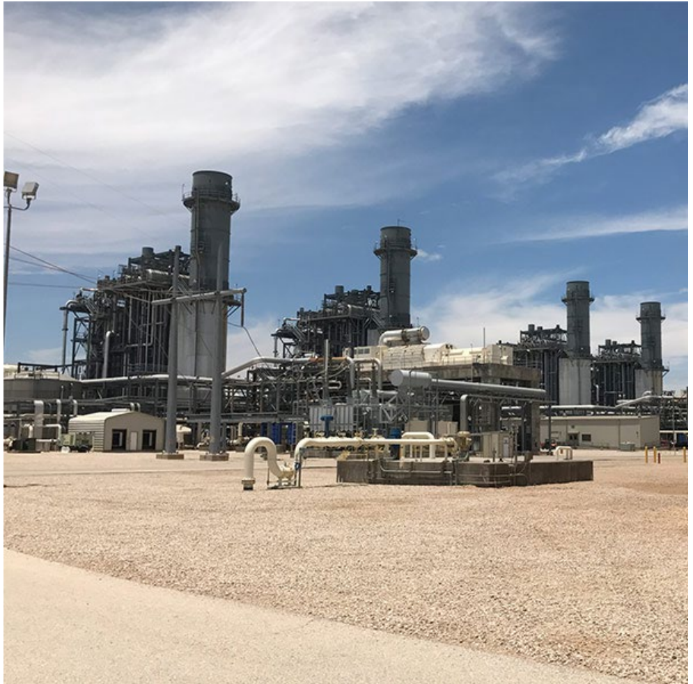
Luminant’s Odessa-Ector gas plant stands ready for possible scarcity pricing later this summer. | Luminant
