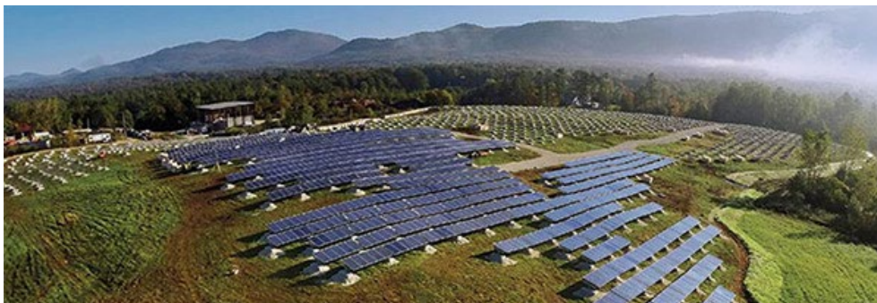
Green Mountain Power's Stafford Hill Solar Farm in Rutland, Vt., was the first in the region to use battery storage to reduce peak demand. | UVM
