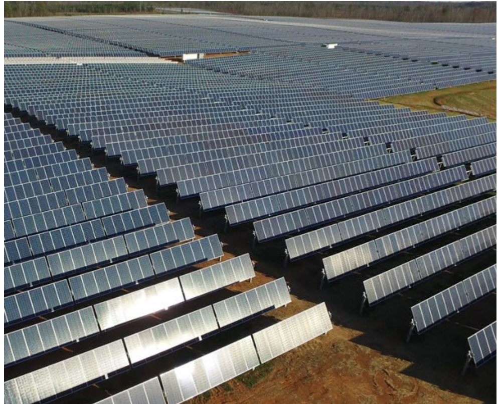
Dominion Energy solar farm in Virginia | Dominion Energy
