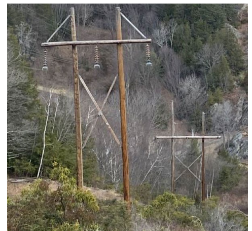
Eversource Energy will spend $38 million to replace conductors and wood poles on its 10.3-mile, 115-kV line between Harwinton and Watertown, Conn. | Eversource Energy
