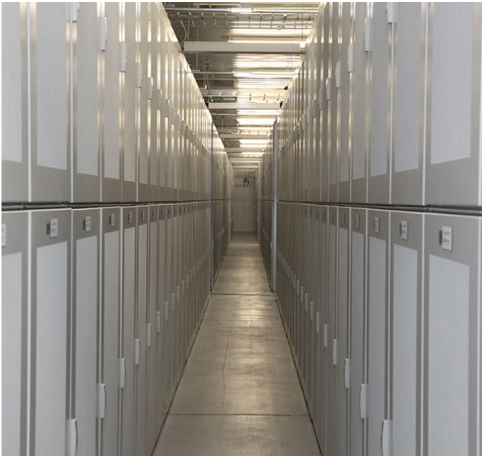
Banks of utility scale battery storage | Southern California Edison
