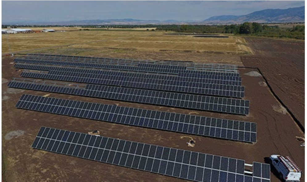
NorthWestern Energy and Bozeman Solar Array | OnSite Energy
