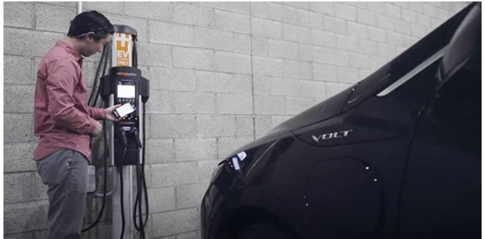
SCE's Charge Ready program installs chargers at multiunit dwellings. | Southern California Edison
