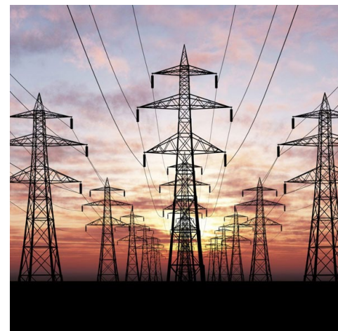
Transmission lines in the WAPA footprint | Southwire
