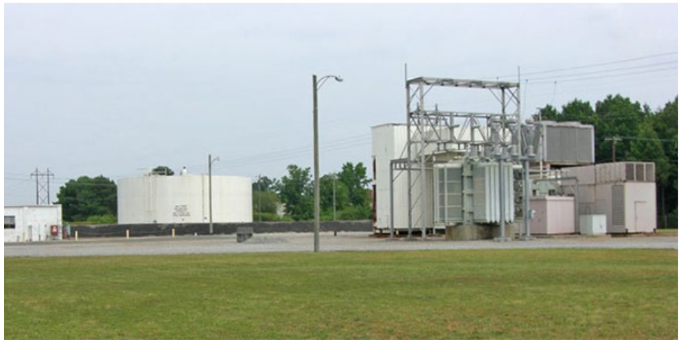
Tasley, a single-unit 33 MW industrial gas turbine that began commercial operation in 1972 in Tasley, Va., is a black start-capable unit. Calpine acquired Tasley in 2010 as part of its purchase of the Conectiv Energy assets. | Calpine
