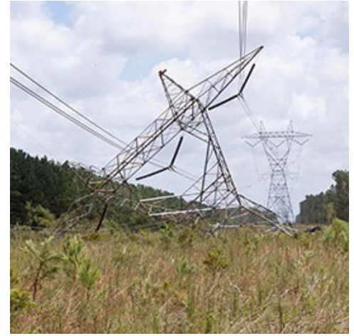
Damaged transmission tower after Hurricane Laura | Entergy
