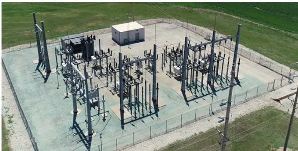
GridLiance substation | GridLiance
