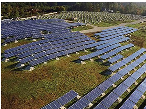
Green Mountain Power's Stafford Hill Solar Farm in Rutland, Vt., was the first in the region to use battery storage to reduce peak demand. | UVM
