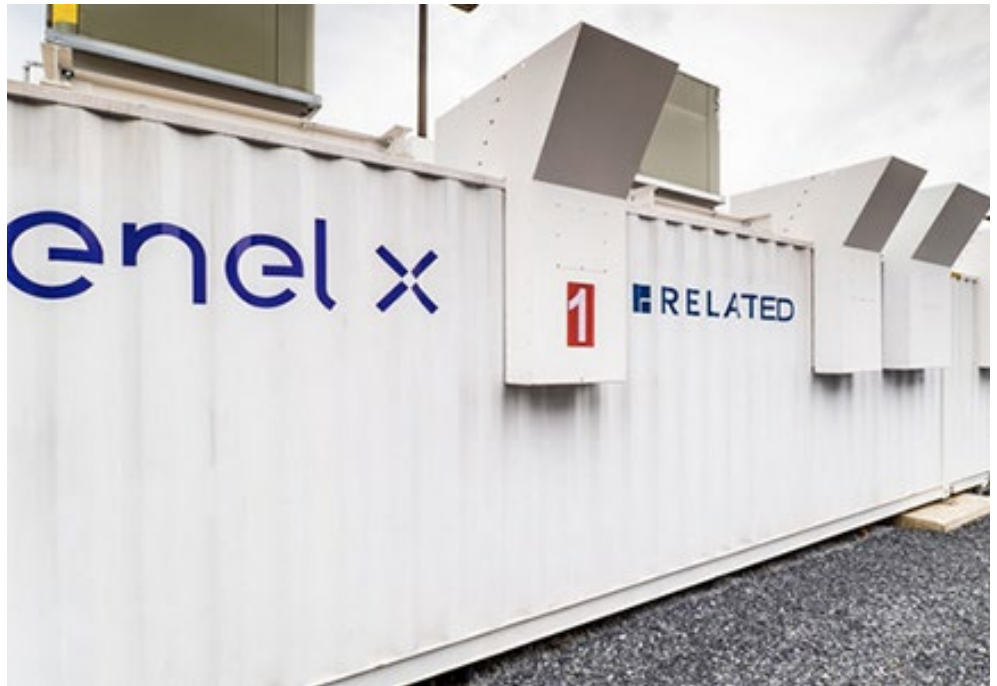
Enel X installed, owns and operates this 4.8-MW/16.4-MWh front-of-the-meter battery system, which was paid for in part by Con Edison via its Brooklyn Queens Demand Management Program. | Con Edison
