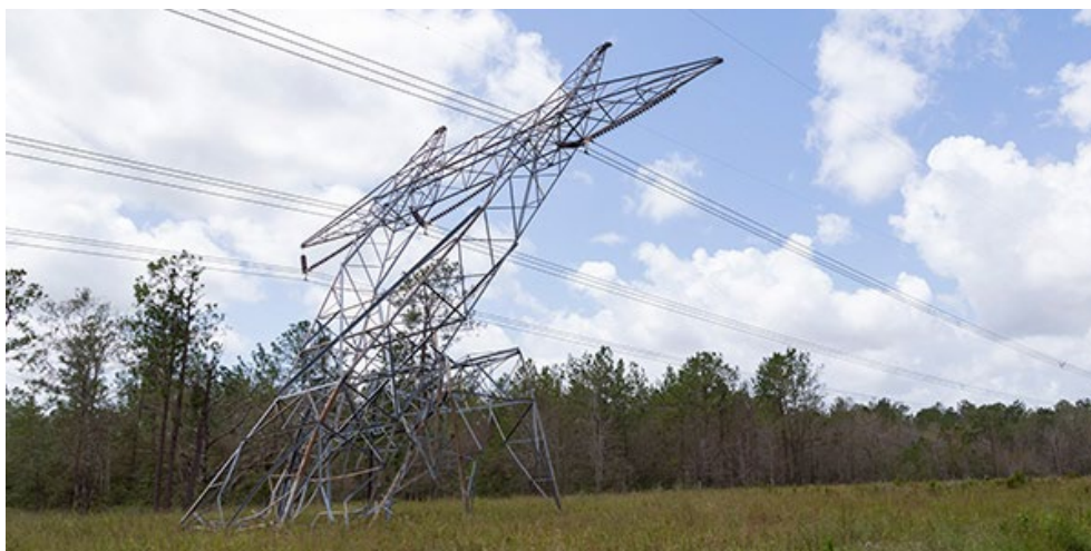
Damaged transmission infrastructure caused by Hurricane Laura | Entergy
