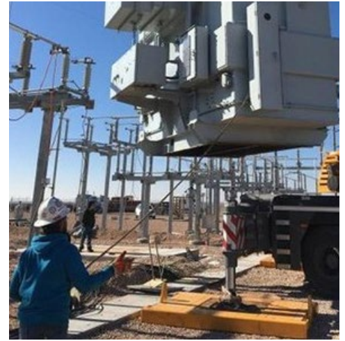
Workers install a transformer on Tri-County Electric Cooperative's Panhandle Substation, part of a transmission upgrade project with GridLiance. | Tri-County Electric Cooperative
