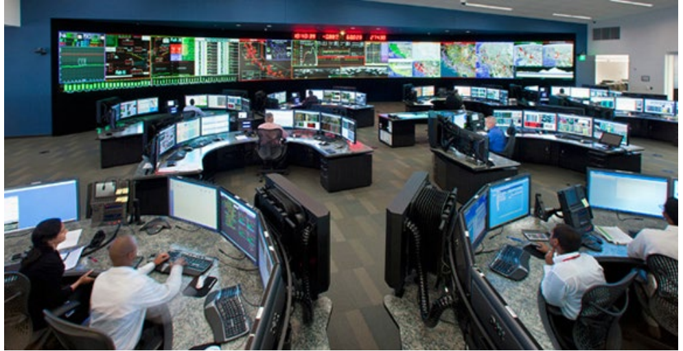
CAISO's control room in Folsom, Calif. | CAISO
