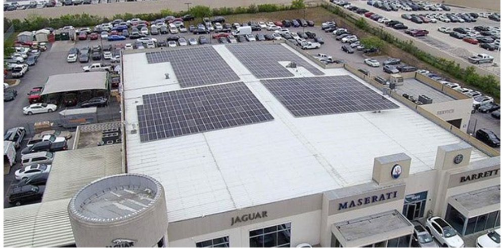
Freedom Solar Power's 214-kW solar array at a car dealership in San Antonio | Freedom Solar Power
